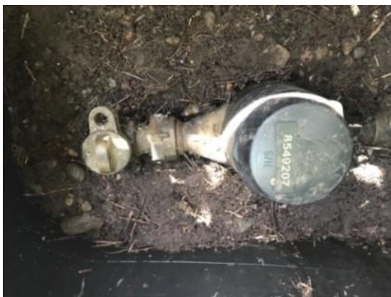
Figure 2. Water shut-off valve, closed
